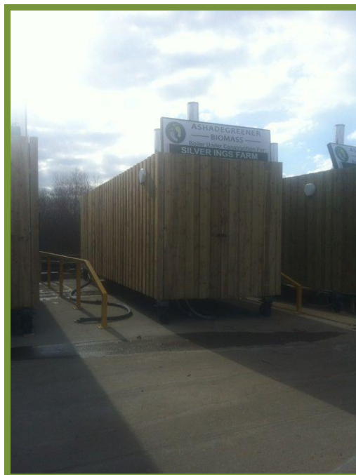
Fig 6 – Containerised biomass boiler
