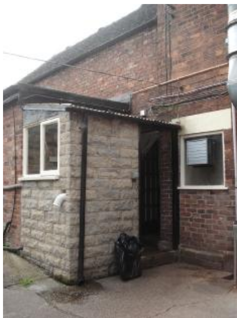
Existing lean-to lobby – Uncertain if permissions have previously been sought.
