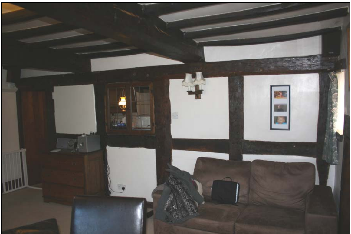
13. Timber-framed wall in wing: top and bottom panels on right contain wattle-and-daub infill
