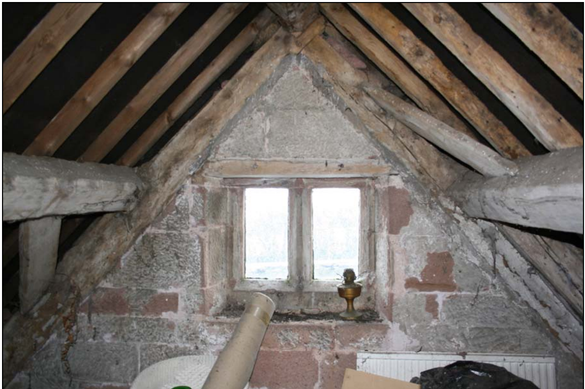
7. Attic of crosswing, showing windbraced truss embedded in gable wall, indicating stone cladding of a box-framed building
