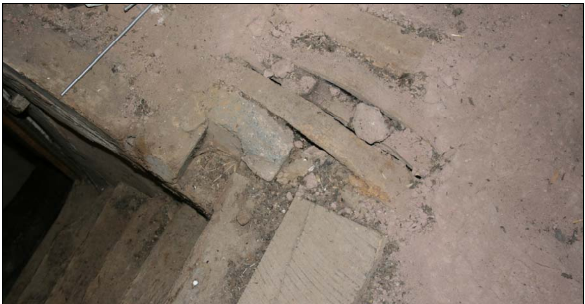
17. Clay floor exposed in attic around landing of staircase from first floor
