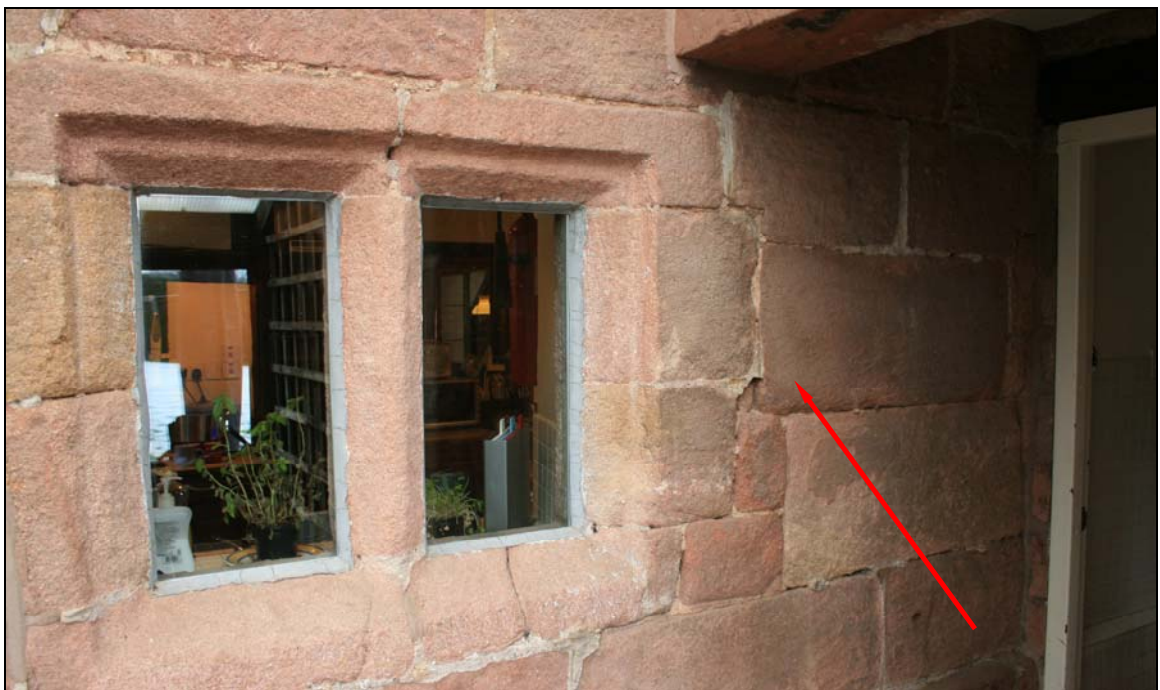
15. Present kitchen window, showing some evidence of rebuilding to right
