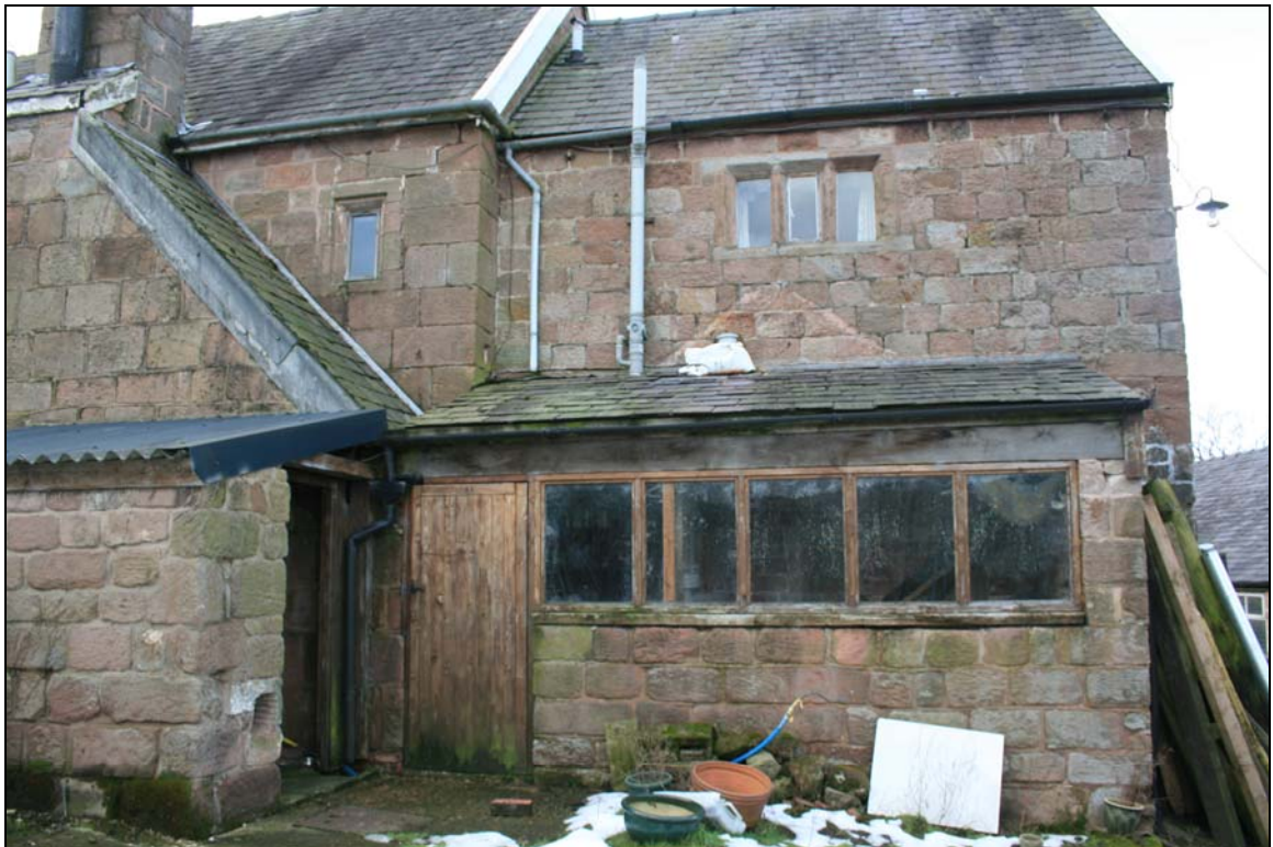
12. Boiler house (left) and ferret house; scarring of gable of former wood store above latter
