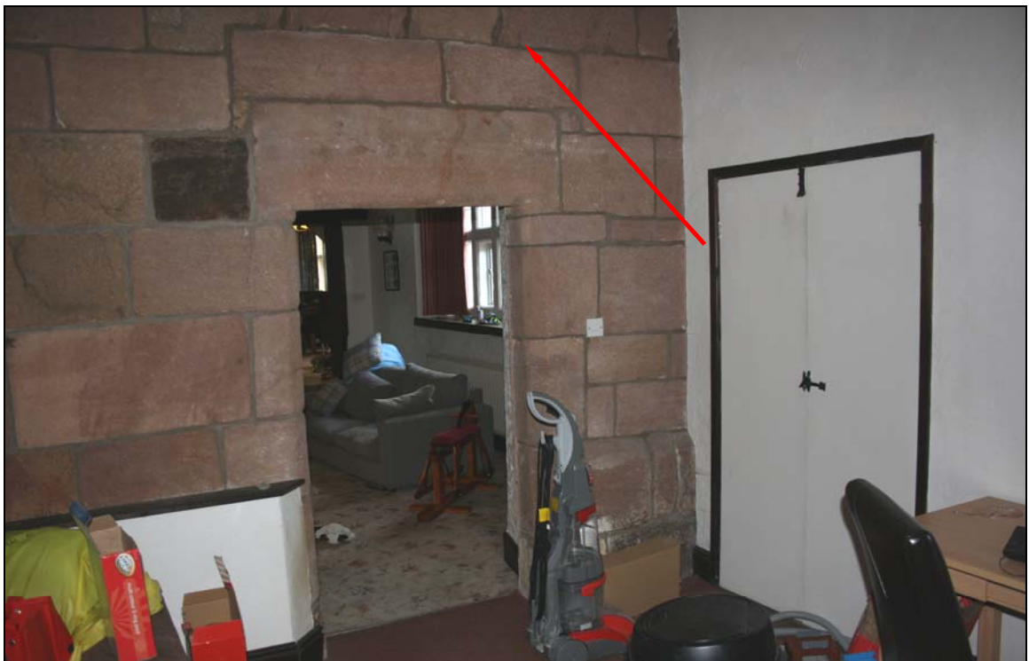
6. Interior of service wing, showing external entrance on right and door to housebody in main range: the latter suggests a cross-passage in the predecessor of the service wing. Joists housings of possible former porch indicated
