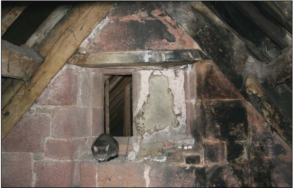
5. Partly blocked window in attic gable indicates predecessor of present service wing was of lower height than the main building
