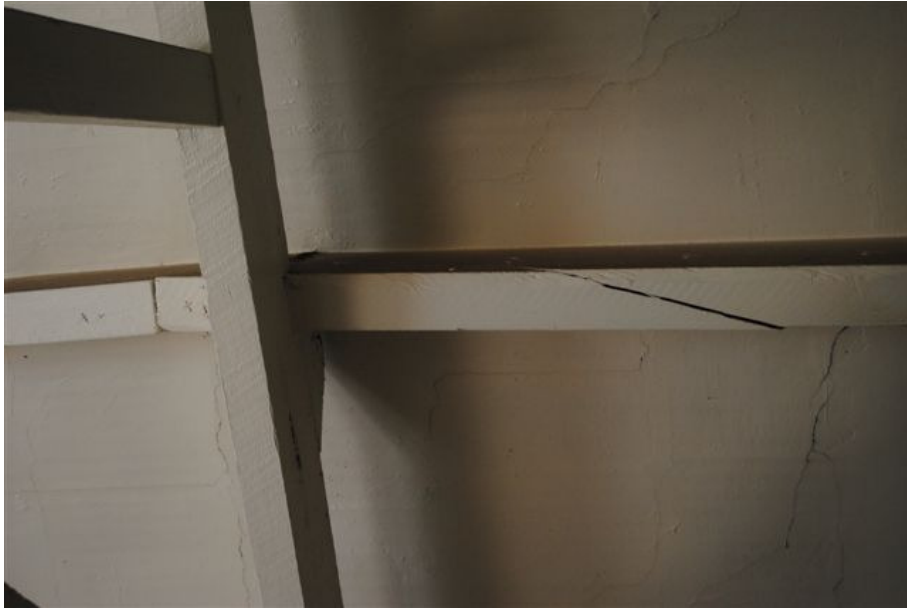
Photograph No. 19: View on roof purlin to West Building showing displaced joint
