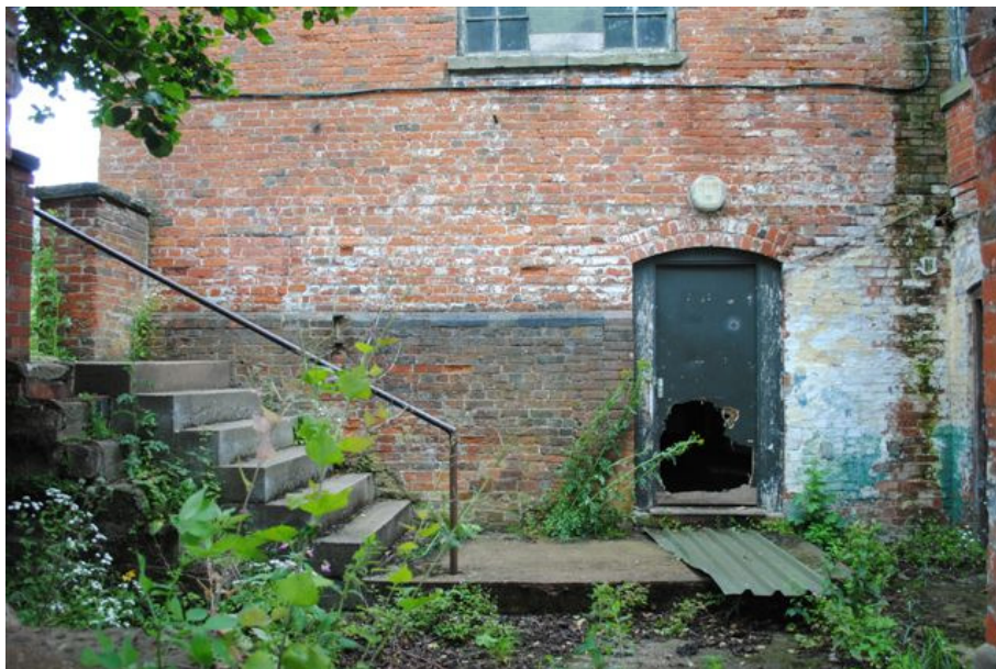
Photograph No. 6: Part View on South Elevation of West Building (lower level)
