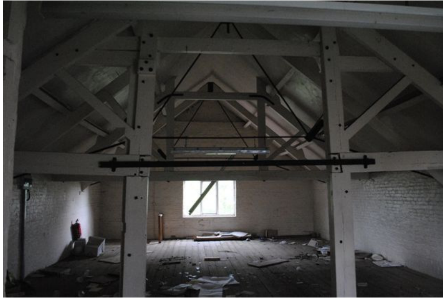
Photograph No. 17: View on Timber Framework supporting Loft in West Building (Note metal horizontal tie bar)
