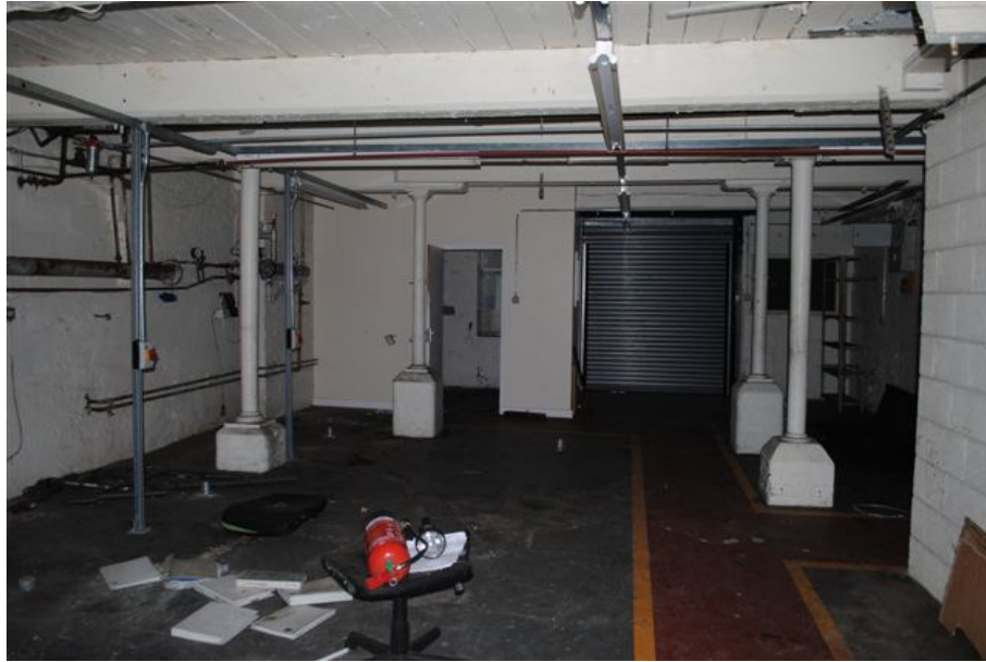
Photograph No. 9: View inside Ground Floor Room of West Building (Note columns supporting first floor beams)
