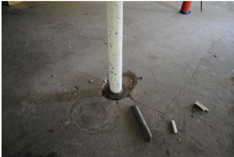
Photograph No. 12: Part View on First Floor of West Building showing screed failure and unfixed base of steel post
