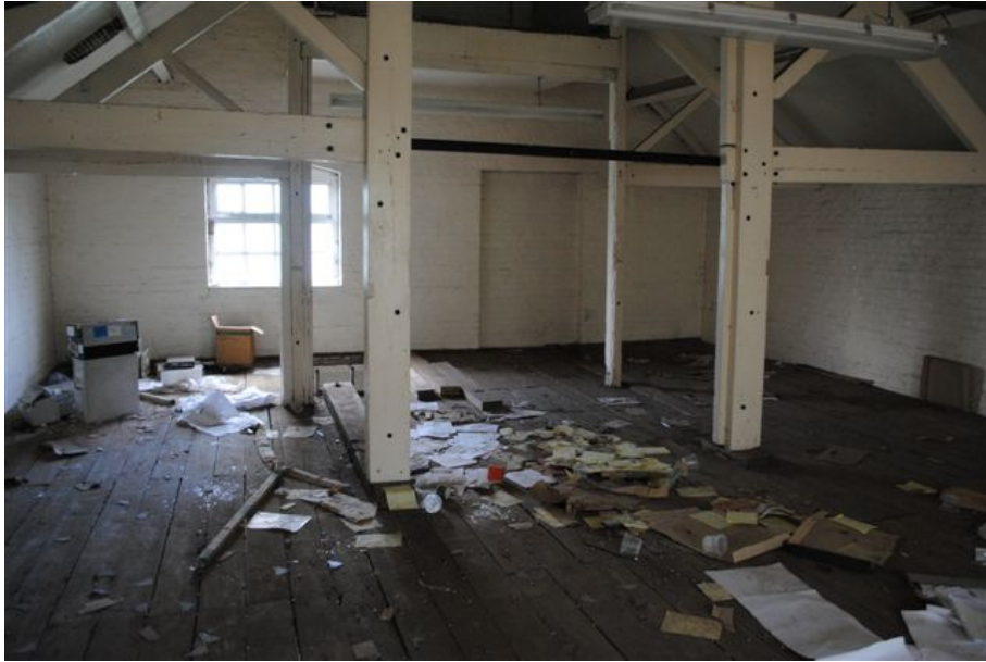
Photograph No. 13: View inside Second Floor of West Building showing timber framework to Loft
