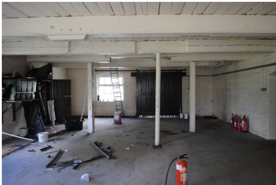
Photograph No. 10: View inside First Floor of West Building (Note columns/post and cut outs in face of primary timber floor beam)
