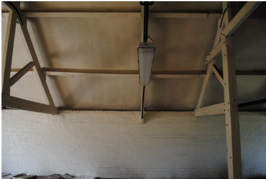
Photograph No. 18: View on underside of roof slope to West Building (Note deflection in purlins)
