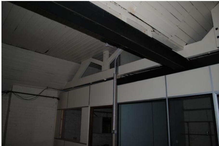
Photograph No. 8: Part View on underside of roof to the East Building
