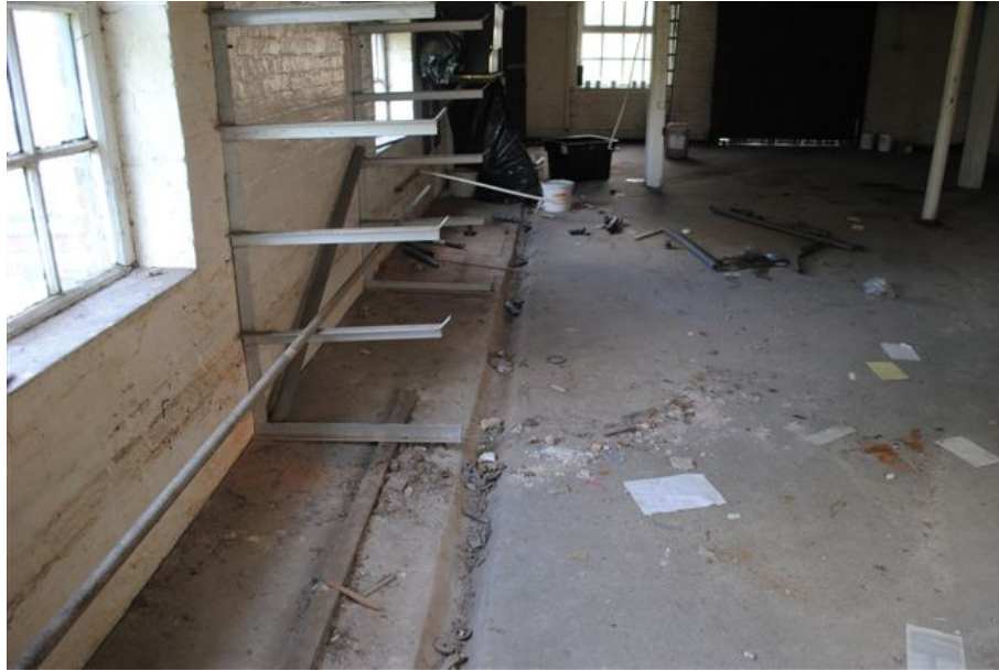
Photograph No. 11: Part View on First Floor of West Building (Note cement based screed and open drain channel)
