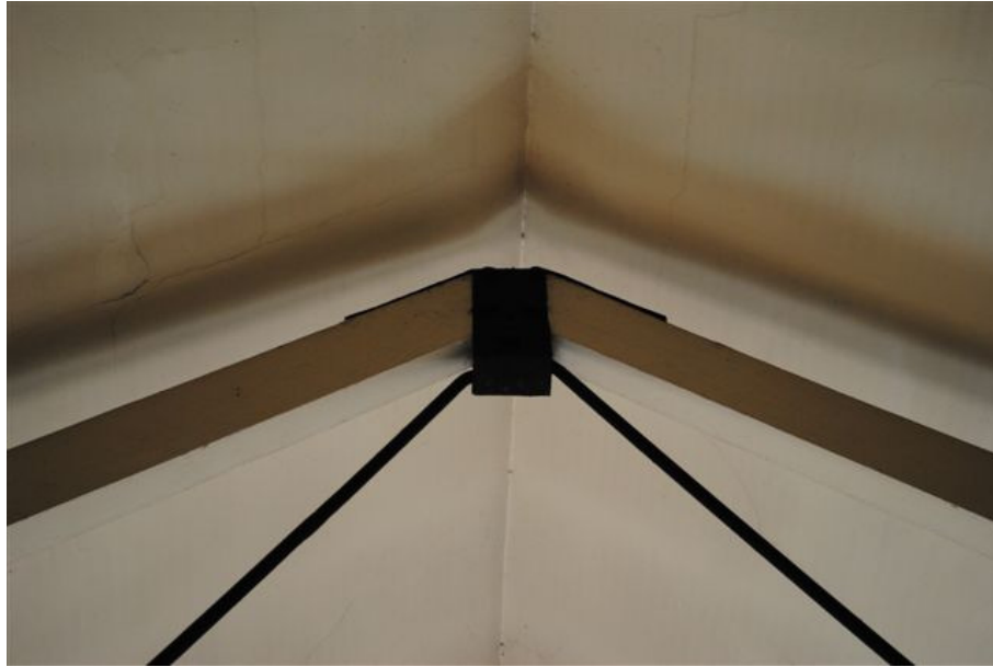
Photograph No. 15: Part View on Composite Roof Truss to West Building (Note gap between apex and underside of ridge)
