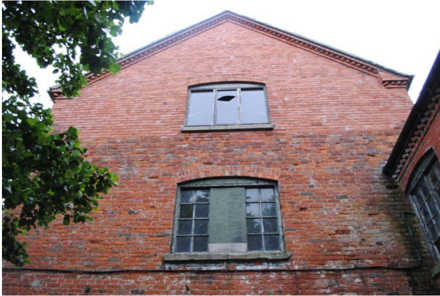
Photograph No. 5: Part View on South Elevation of West Building (Upper level) (Note change in brickwork above first floor window cill)
