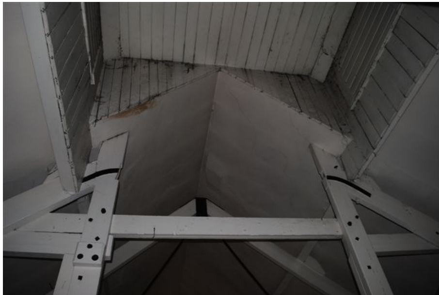
Photograph No. 16: View on Timber Framework to underside of Loft in West Building
