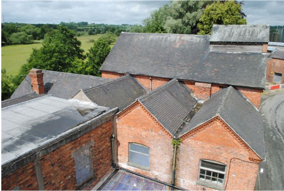
Photograph No. 1: Aerial View on Engineering Offices (Note: Engineering Stores Building in the foreground to the left and the roof of the Cottage in the background to the left)
