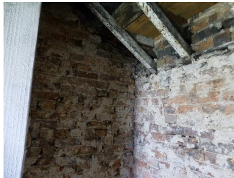
Fig.3 Inadequate bonding between external wall and internal loadbearing wall and brickwork built off original timber soleplate
