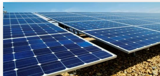
PV System components
