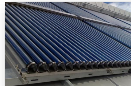
Example of Solar Thermal unit
