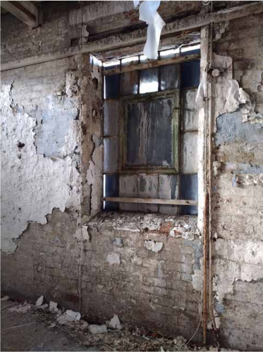
31. Typical example of the condition of the internal wall face - with mutiple layers of paint over lime-wash and trunking.
