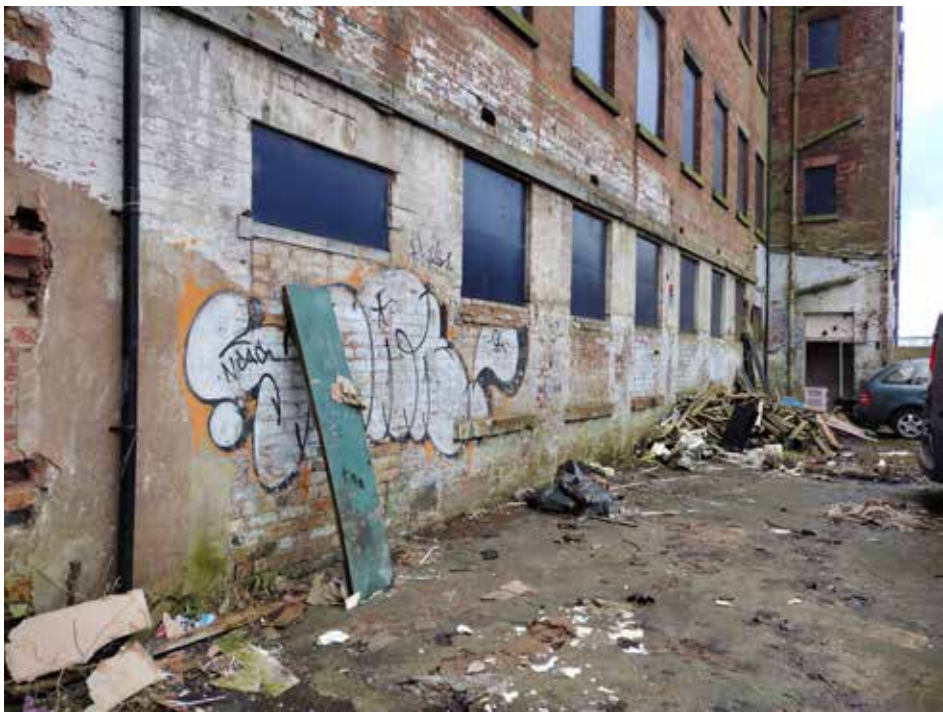
37. The north elevation has suffered from some graffiti and the removal of the rear Boiler House has exposed the former internal wall.
