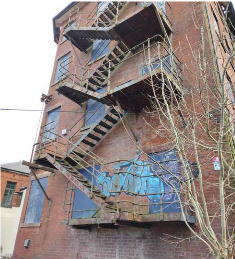
33. The western fire escape staircase is heavily rusted and suspended in mid air, with the bottom flight removed
