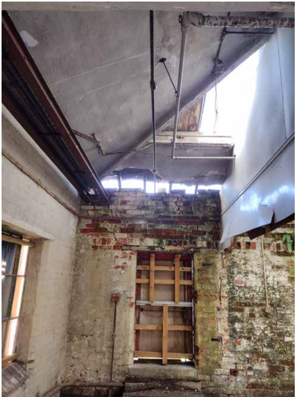
36. The building is not wind and watertight and there are gaps at eaves level over the western elevation, and the eaves masonry is in a degraded condition. This section of the roof is open to the elements, with missing sections of slate and battens, and no sign of a gutter.
