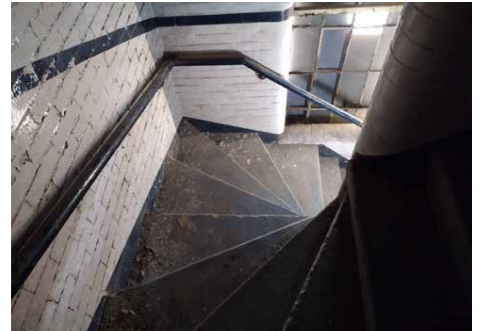
16. Detail of stone winder staircase, with later concrete repair.
