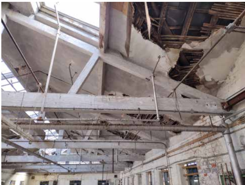
32. Example of the variable condition of the internal roof slope, with missing and damaged sections of lathe-and-plaster.
