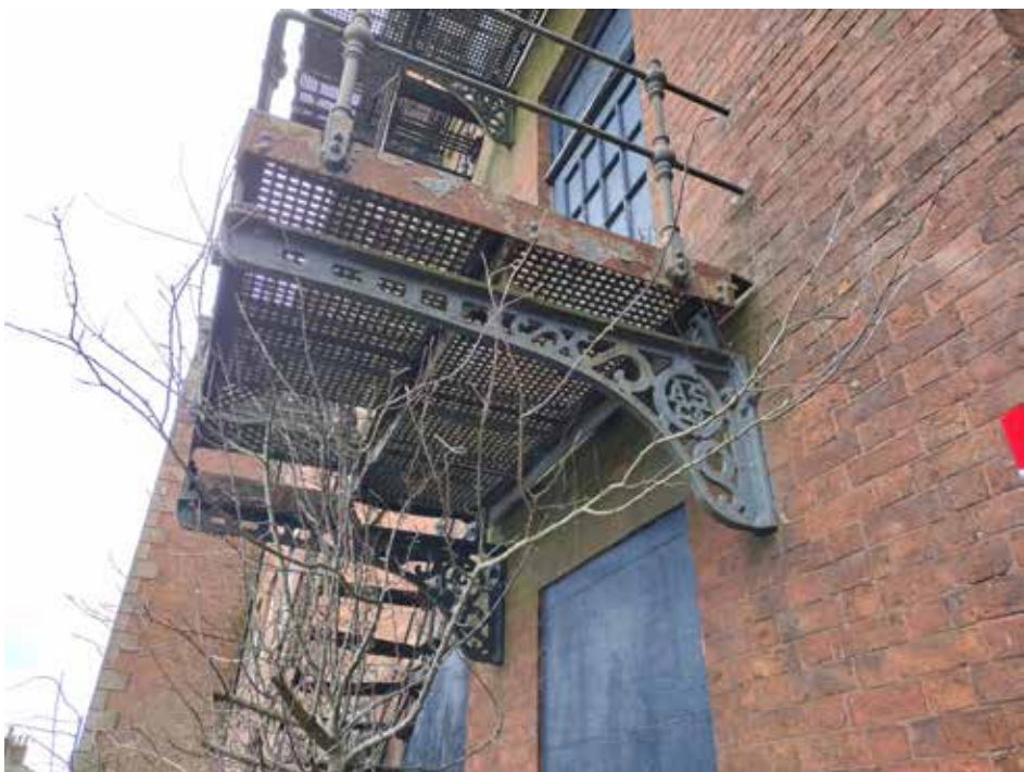
38. The more important cast-iron fire escape staircase is in poor condition, rusting, and needs fully blast cleaning and re-decorating.
