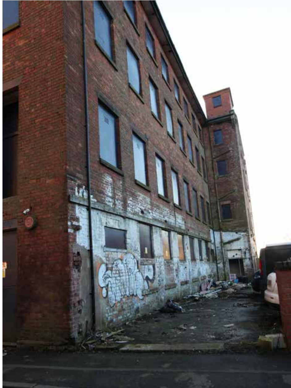
25. View of the rear elevation and yard to Well Street. Removal of the Boiler House and Engine House has left some visible scars which will need to be addressed through sensitive cleaning and repair.
