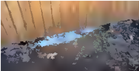
Damp ground above retaining wall at the bottom of Billys croft garden above Leek Old Road, water soaks through to culvert
