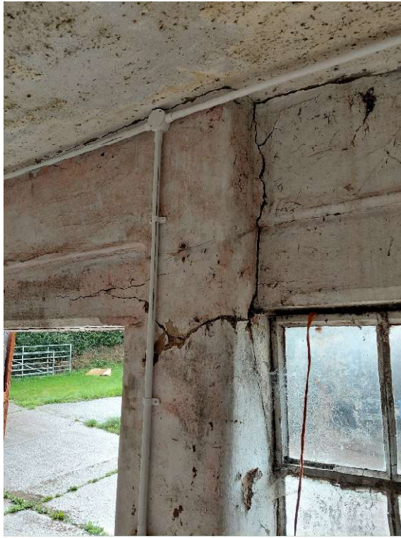
Cracking from lintel
