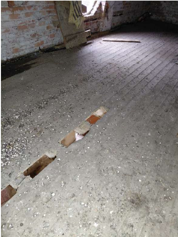
Damaged first floor
