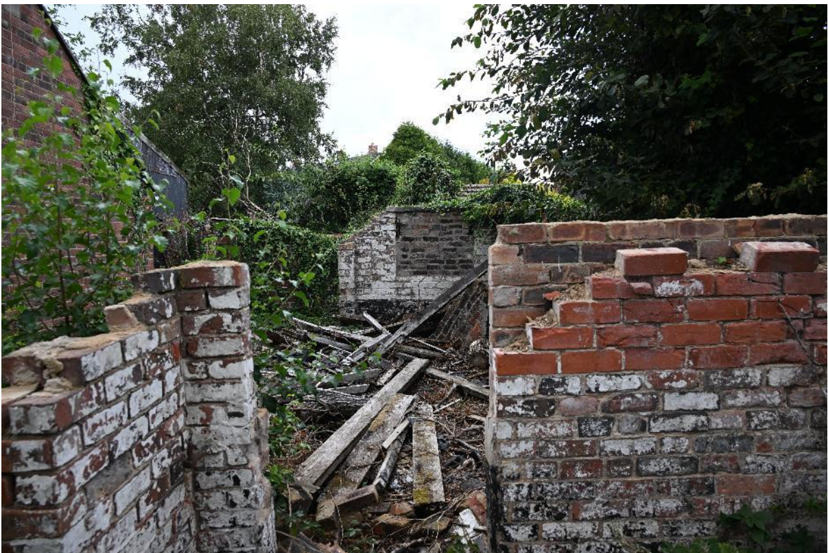
Image 8 Target Building 4 derelict building
