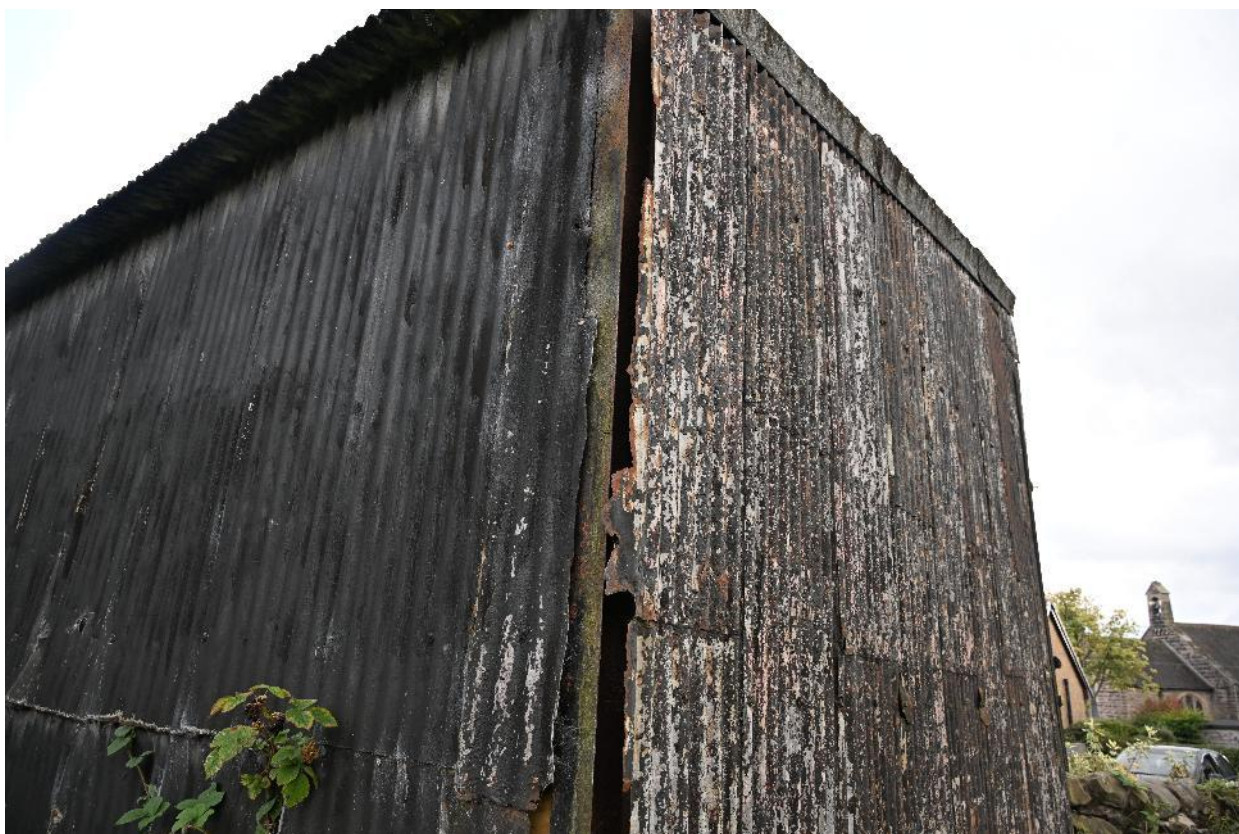
Image 3 Target Building 1 with large gap allowing water ingress
