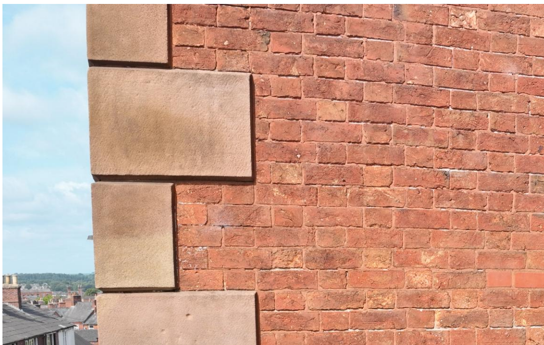
Image 1. Loss of Fired face, coarsening of surface due to previous cleaning.
