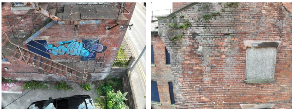
Image 1& 2: Graffiti, salts and atmospheric staining.
