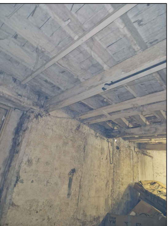
Fig. 6 - Shows the current conditions of the ground floor ceiling, under side of the 1st floor.
