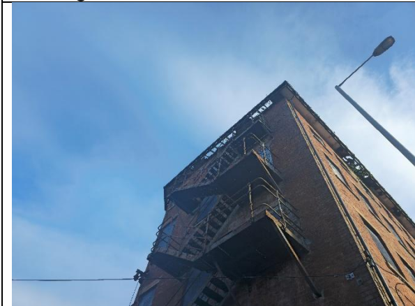
Image 3: Western aspect, visible structural cracks visible in brickwork.
