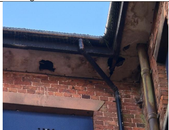
Image 6: Close view of damage soffits, rear central section.
