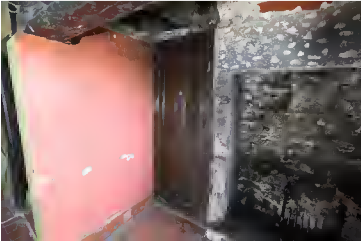
26. 19 th century cupboard within smokehood area. Internal warped shelves to be replaced.
