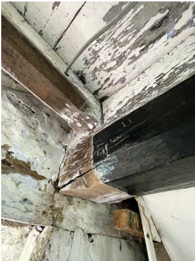
33. Detail of spine beam which has some deterioration and rot bearing onto the internal timber frame and the wall, with test area of steam cleaning to joist.
