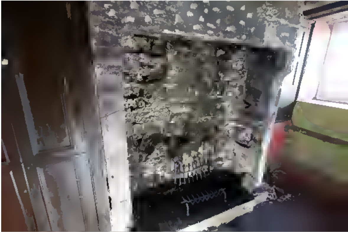
20. Exposed stone jambs and scutched lintel, with shaped jowelled jambs. The detail is typical of the mid 18 th century. Stone masonry wall to rear is coeval with the 18 th century hearth but is in very poor condition. Rather than carry out local rebuilding, a hand-made brickwork backing is proposed to the hearth, using a narrow, 2-inch slop-moulded brick, which will also provide on its top ledge a space for fixing a steel baffle plate for the log burner.
