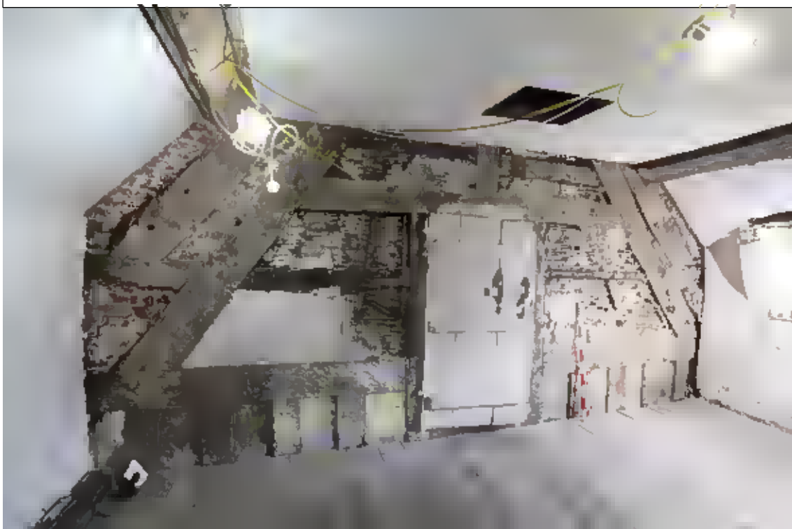
7. Closed truss with wattle-and-daub infill of 1624 and original doorway, largely intact but needing repair.
