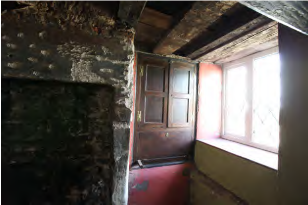
23. 18 th century china corner cupboard with writing desk and altered fire window. Soffit needs local reinstatement of plasterboard and plaster skim.
