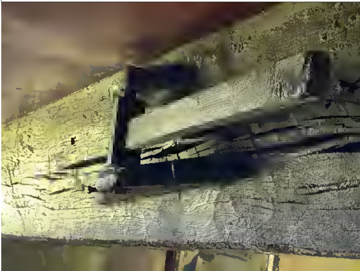
27. Oak bracket for pot hanger to back face of bressummer (in-situ – probably 17 th century).
