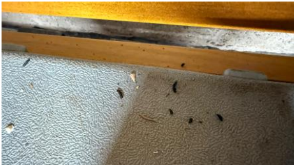
Image 5: small number of bat droppings behind the northern gable wall inside the building
