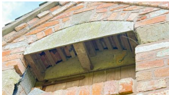
Image 4: potential access points for bats in the gable wall of the building, above the bricked-up window
