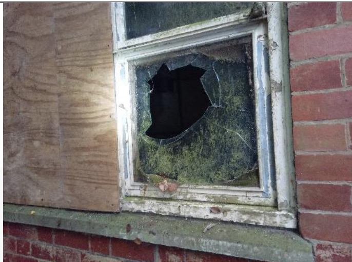
Smashed window along the north elevation.
