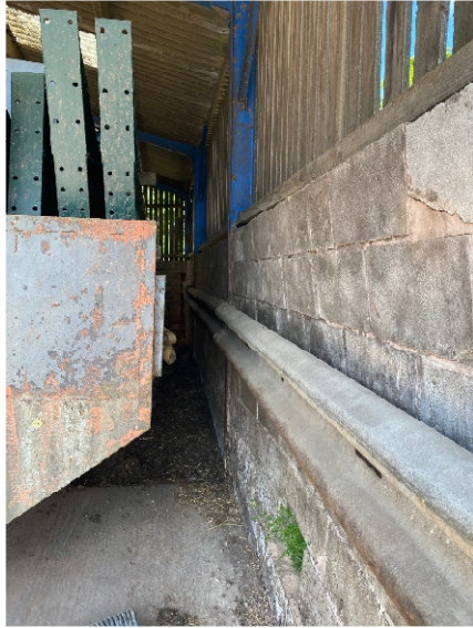
Bay #1 – Internal Elevation note: bowing in blockwork due to historical vehicular impact
