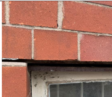
Photograph showing deterioration of corroded lintels and cracking caused to adjacent brickwork.
