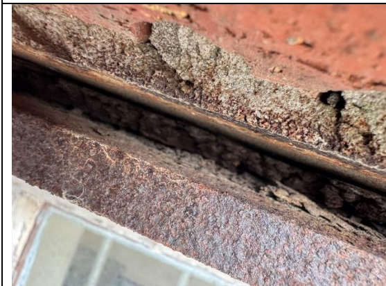
Photograph showing deterioration of corroded lintels.
