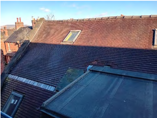
Photo 13: Missing tiles, board, and lifted ridge tiles on the west elevation of B2.
