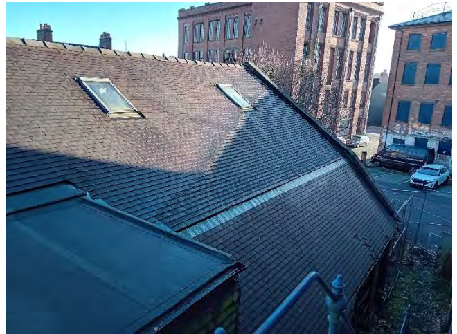
Photo 14: Slipped tiles and lifted ridge tiles on the west elevation of B2.
