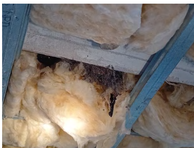
Photo 20: Deceased bird present in the insulation in B1.
