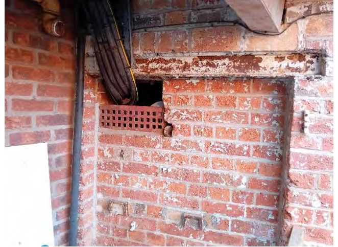
Photo 8: Gap in the grating on the south elevation of B1.
