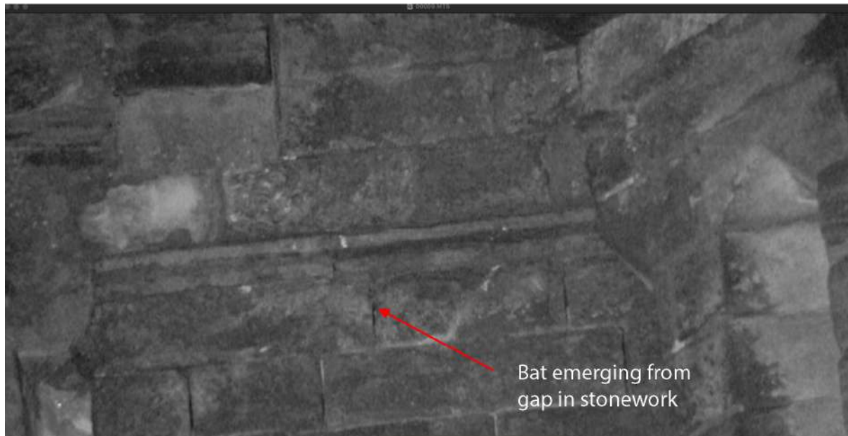
Image 6: red arrow points to bat emerging from narrow gap between stonework on eastern side of apse during the survey on 16 th September 2024
