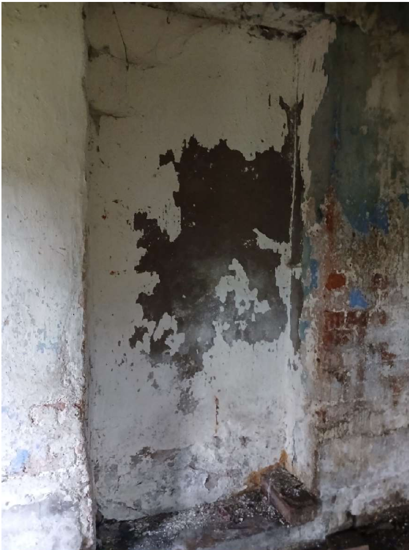
Figure 1 – Blocked internal door from utility
