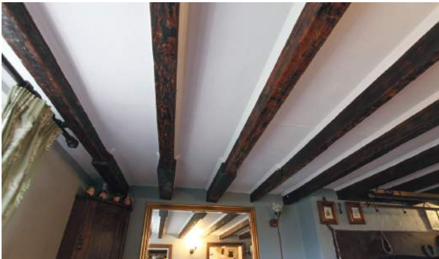
23. Ceiling joists to corner of Dining Room. These have been extended and / or repaired. The home owner says that a blocked doorway was found in this wall when the gable wall was re-plastered and these cropped joists may either reflect the location of a former internal lobby or the location of a former staircase.
