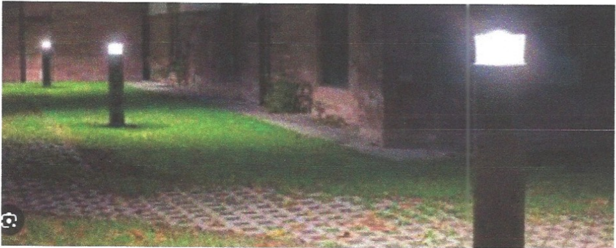
12watt LED bollard lighting
