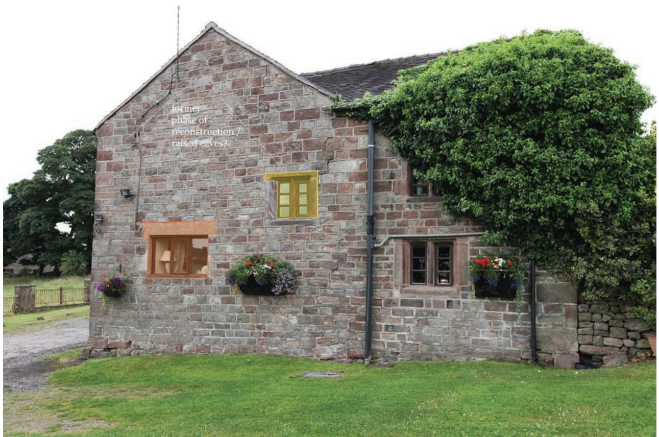
Pl. 8 yellow highlighted masonry dates from the 1992 repair, whilst the orange highlight is a 20th century alteration
