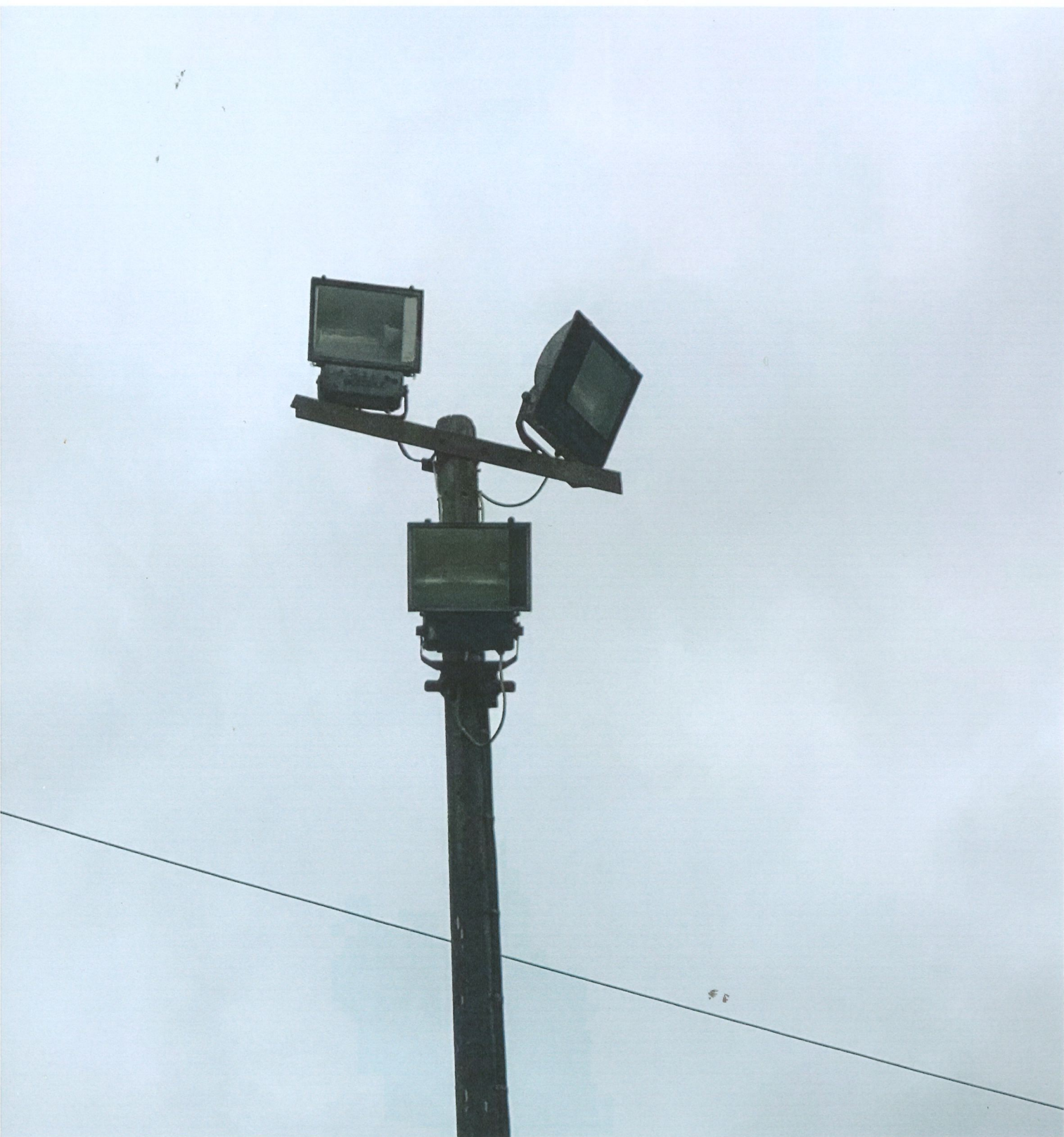
THREE LIGHTS ON EACH OF THE OL POSTS AT 8 METRES.
