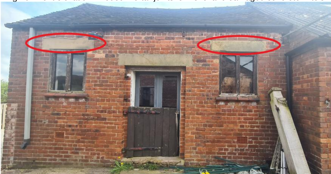
Fig 11. Left hand side of front elevation. Weathered face to stone lintels.
