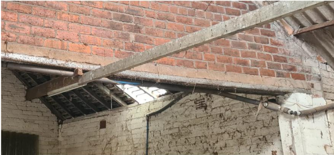
Fig 16. Internal view of bowed rear external wall.
