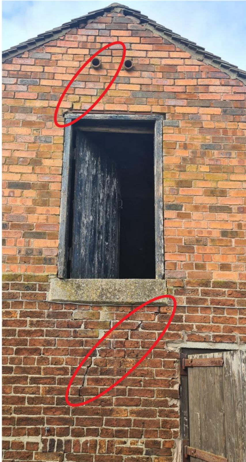
Fig 5. Fine stepped diagonal cracks above and below doorway to rear elevation.
