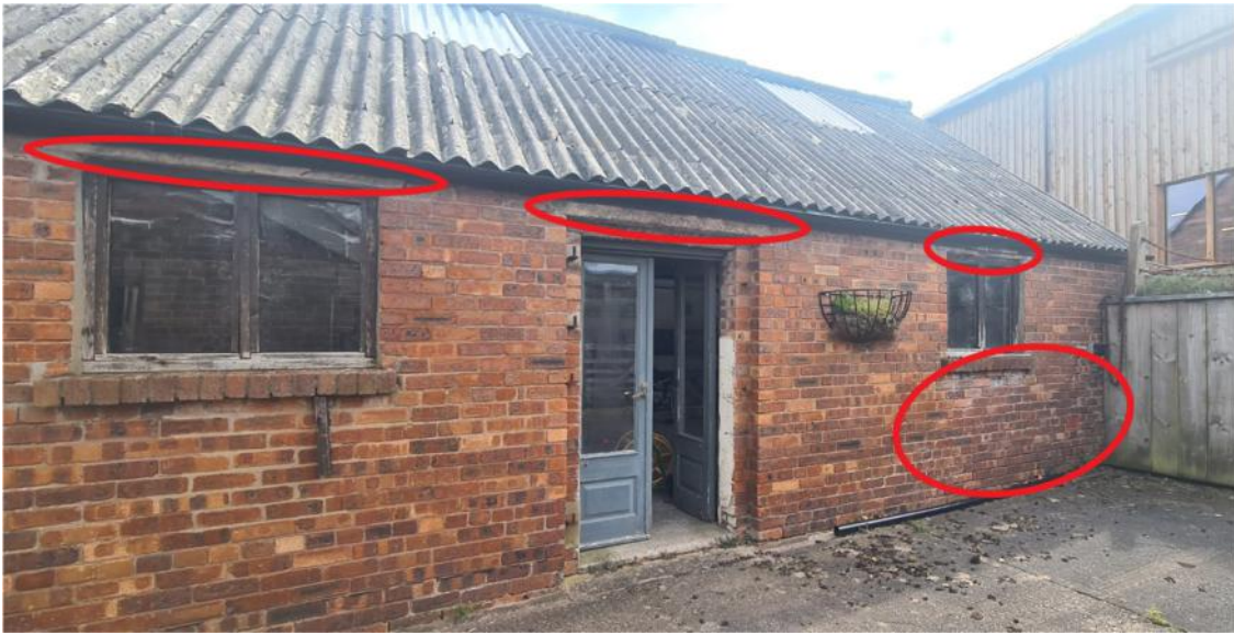
Fig 10. Front elevation. Eroded mortar joints low level and damaged concrete lintels.
