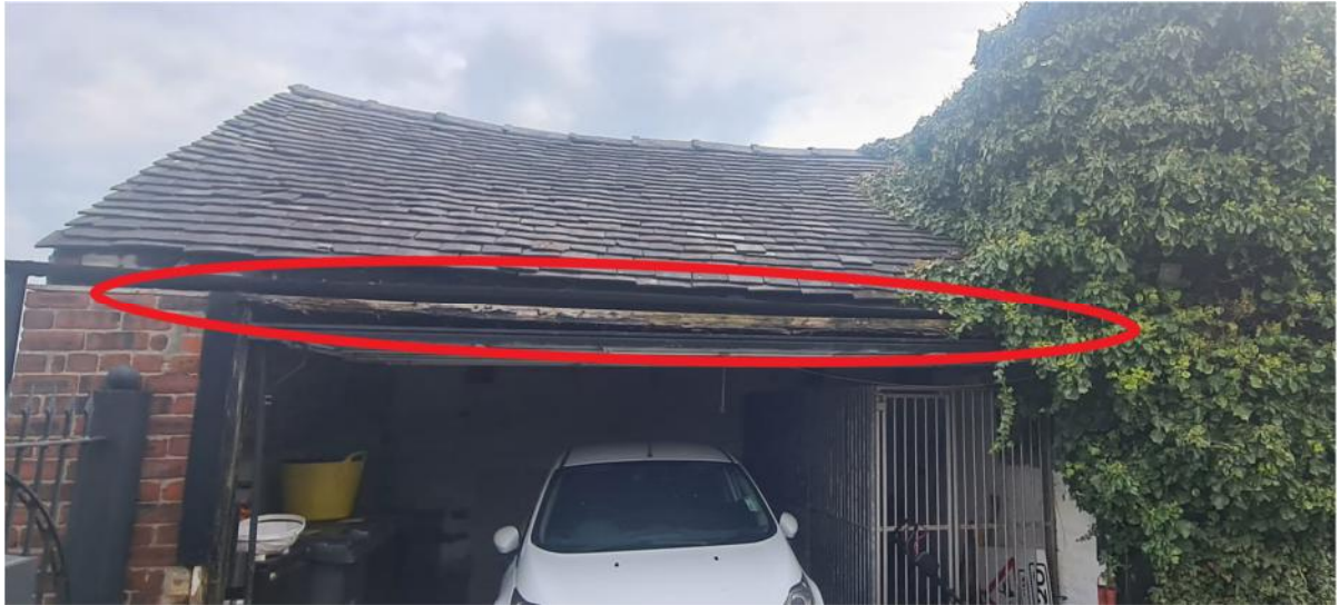
Fig 3. Front elevation where lintel has deflected and should be replaced (By CATNIC or similar approved).
