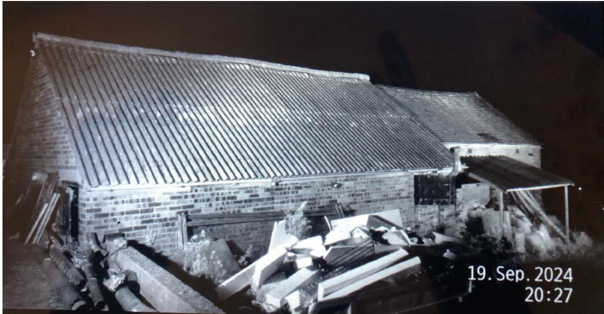
Photo 7: NVA image covering rear east facing roof pitch of B2
