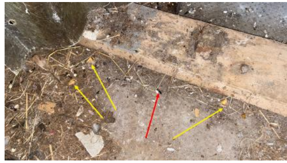
Photo 6: Red arrow points to bat dropping and yellow arrows point to discarded moth feeding remains in B2
