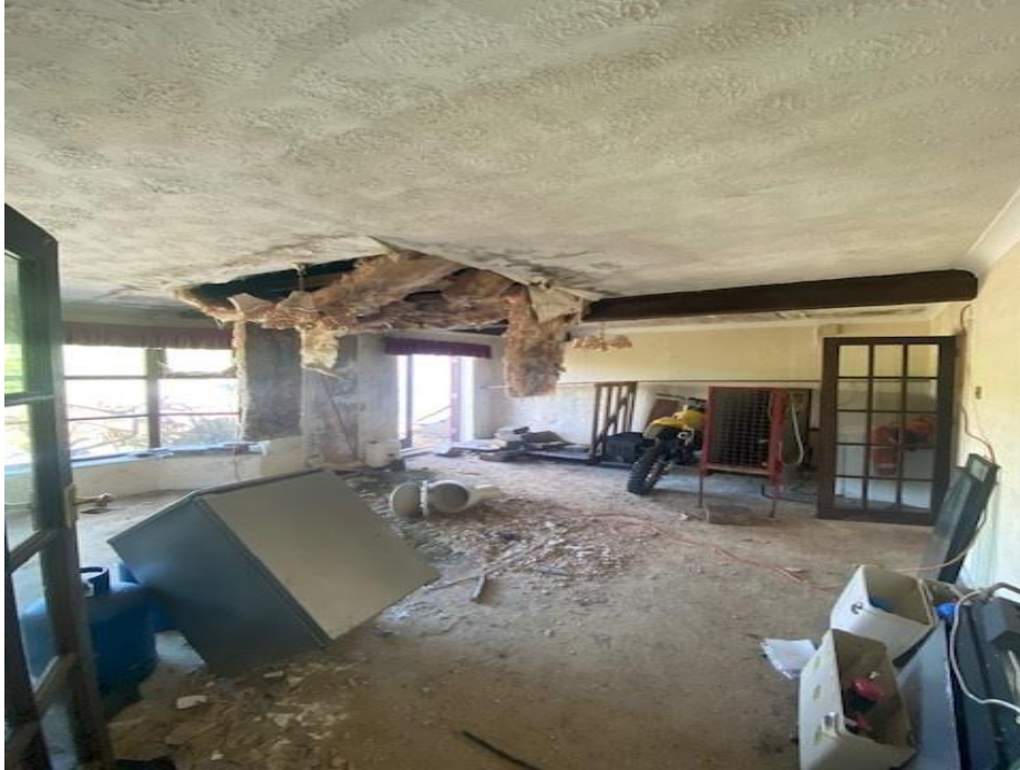
Figure 7. View of living room with partially collapsed ceiling (Grid ref SK 04954 42061)
