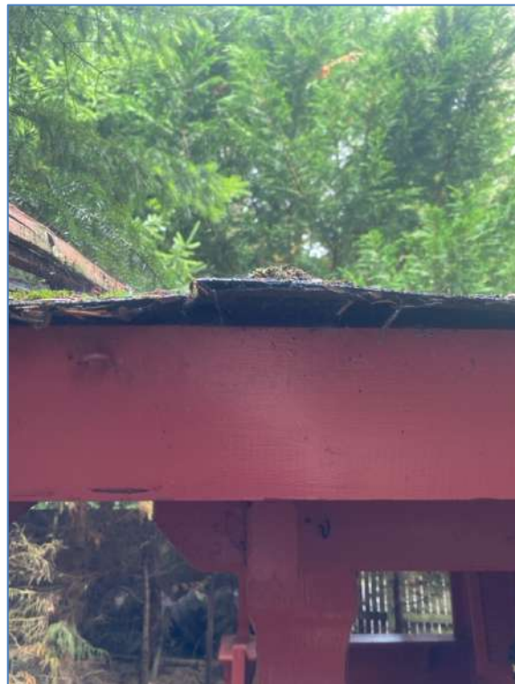
Figure 7. Lifted roof felt
