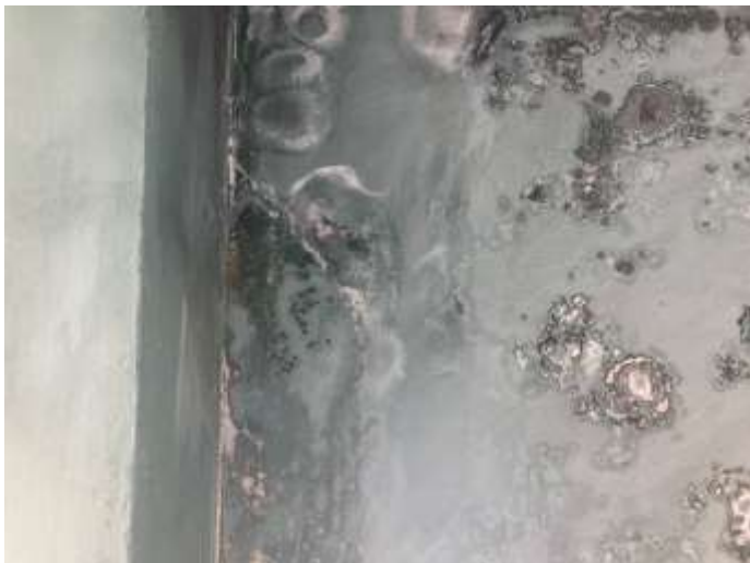
Internal wall damp (WGY 2024)
