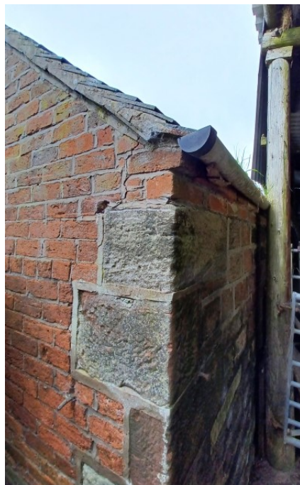
Photo 4: East / North Elevation showing corner (crack to mortar)
