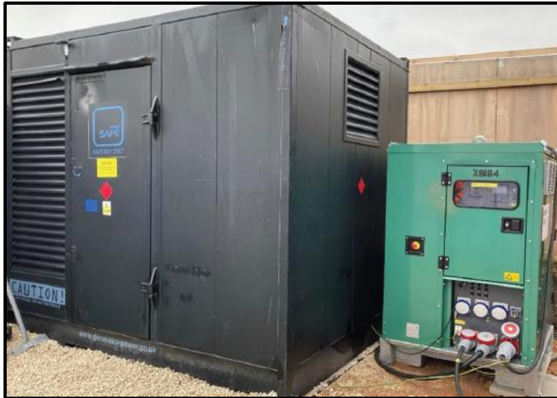
Standard containerised generator with 45KW battery pack
