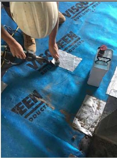
Hole found remediated on site
