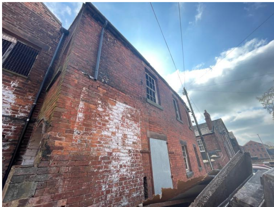
Photograph 3: West facing aspect of Area A (bow in wall)
