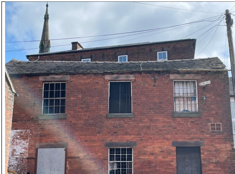
Photograph 1: West facing aspect of Area A (bow in wall)
