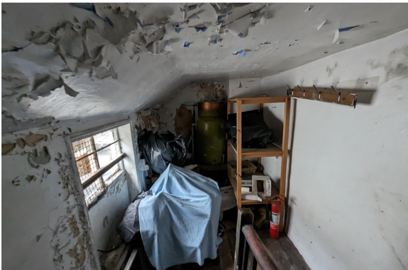
Figure 7: First floor (rear), the building is in very poor condition and a full renovation is necessary.
