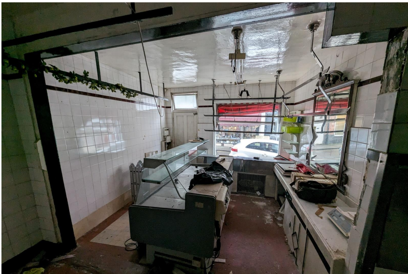
Figure 5: Ground Floor (front) condition; the building is not suitable for re-use without a full phase of renovations.
