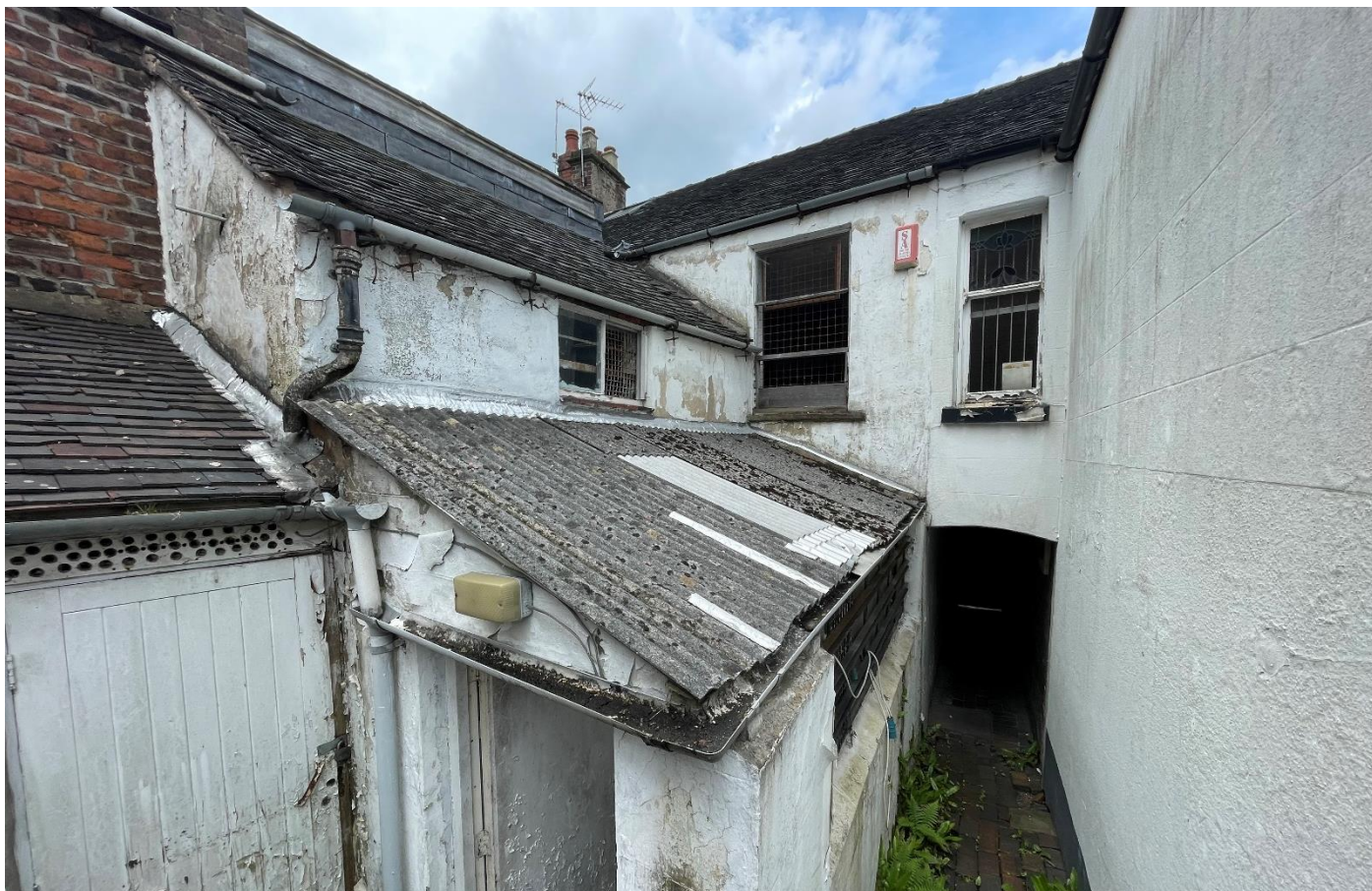
Figure 2: The rear Elevation and shared access. The property does not have weathertight windows and the roof requires replacement.
