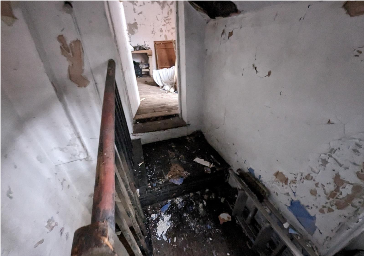
Figure 8: First floor condition is very poor; the roof is leaking in, and the ceiling has collapsed.
