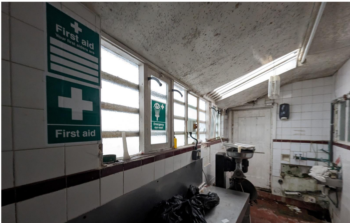
Figure 6: Ground floor (rear); the ceiling has mould spots and has partially collapsed, this requires replacement.
