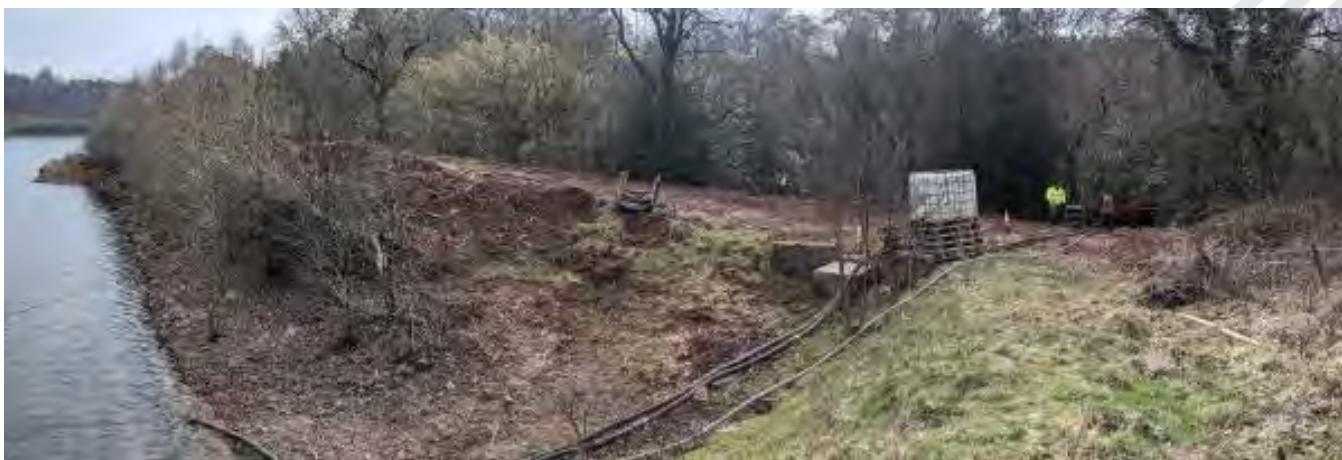
Figure 8-5: Natural Saddle, outfall structure and siphons – including header tank for priming siphons (adapted from Mott MacDonald (2021))
