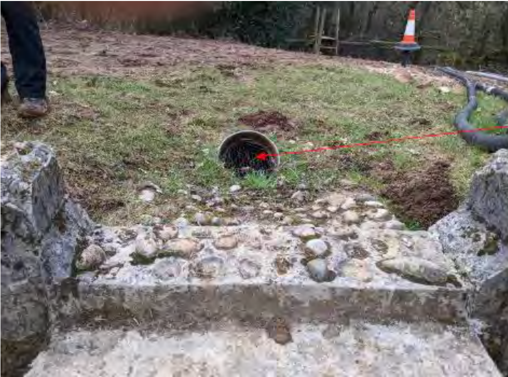
Figure 8-7: Outlet pipe (adapted from Mott MacDonald (2021))
