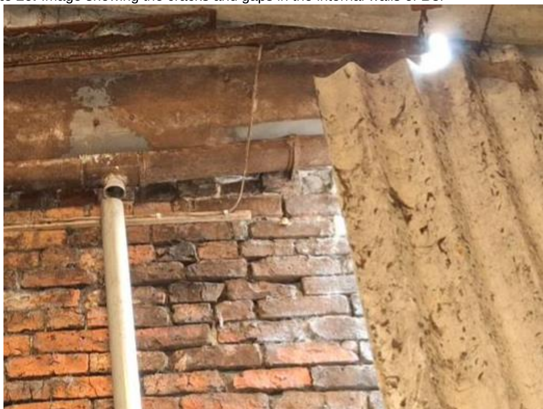
Plate 26: Image showing the cracks and gaps in the internal walls of B5.
