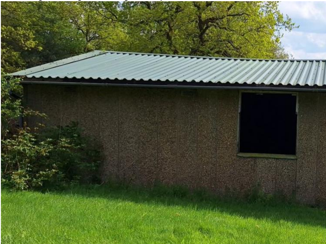
Plate 30: Image showing the missing windowpane on the northern elevation of B7.
