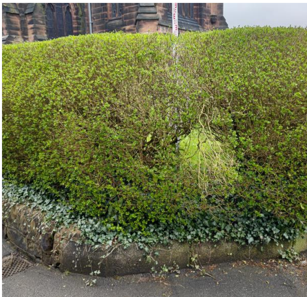
Figure 2 – Hole in existing hedge rendering the school site accessible to intruders.
