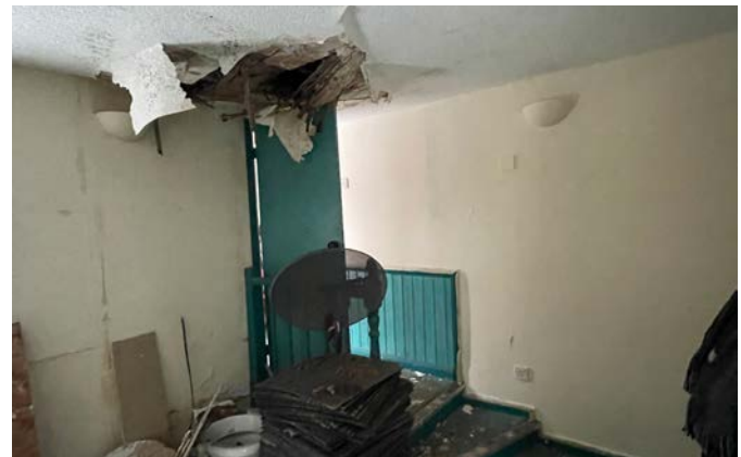
Existing condition inside of the house to be made good and habitable.
