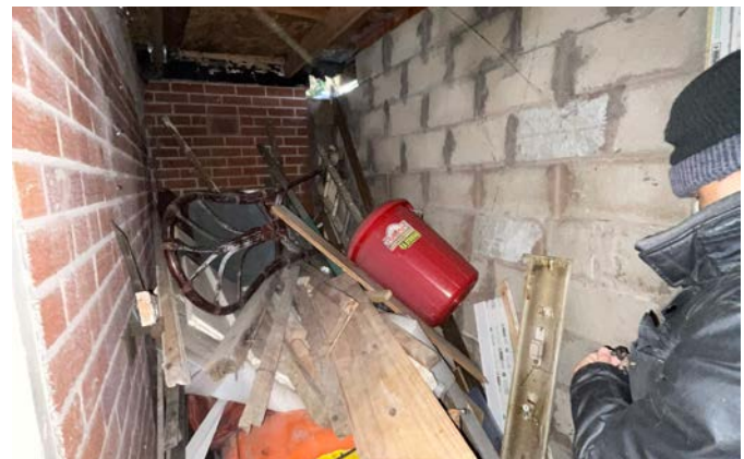
Existing condition inside of property to be made good and habitable.
