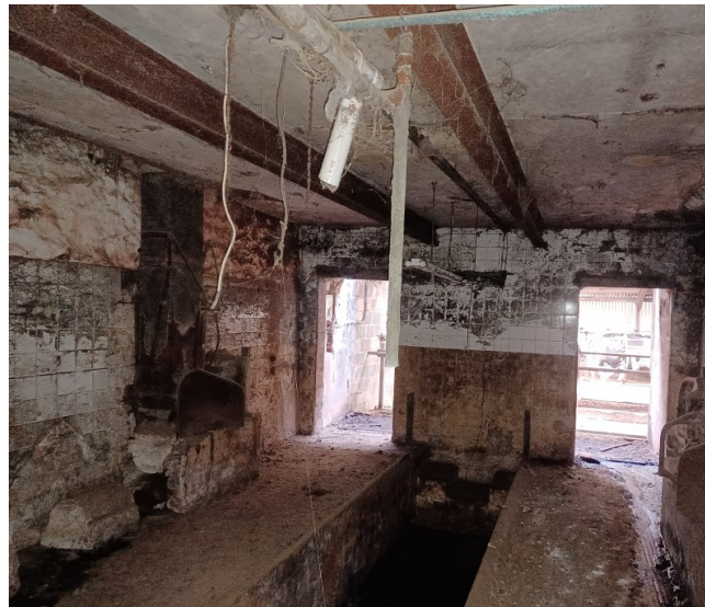
Photo 7: Ground floor milking parlour
