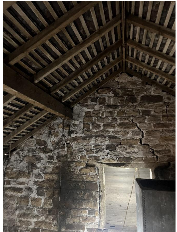
Lintel Failure Sections B & C
