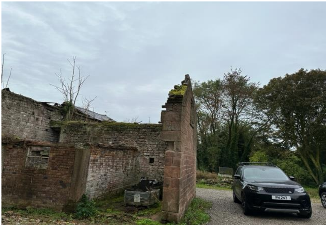
View of north west gable wall – note wall is plumb apart from a small section at the ridge line.
