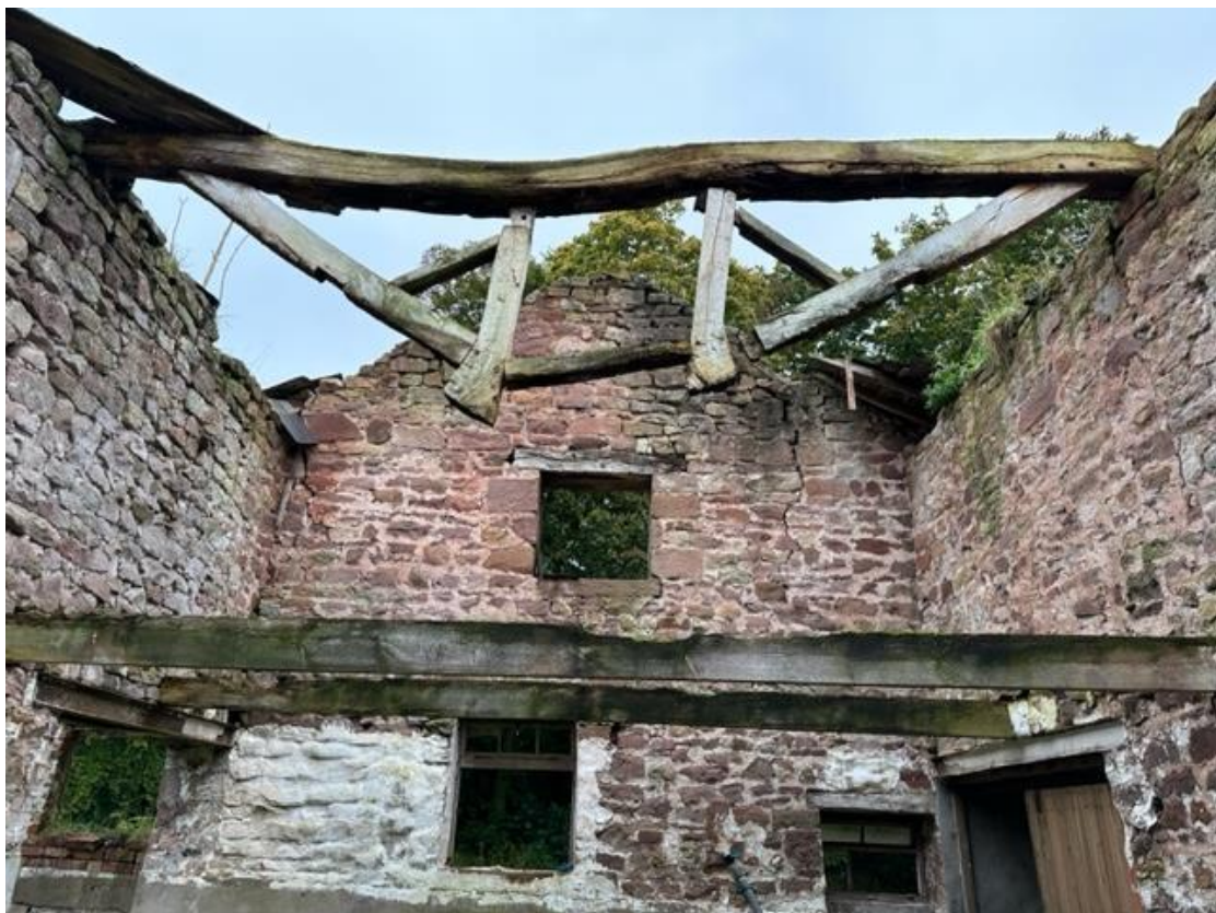
Original roof and floor structure is largely missing – however, this would ordinarily be replaced as part of any renovation to meet modern building regulation standards.
