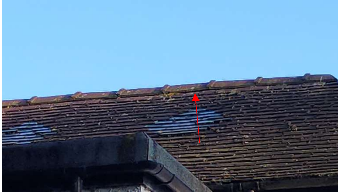
Plate 3: Showing raised ridge tile potential bat access point.
