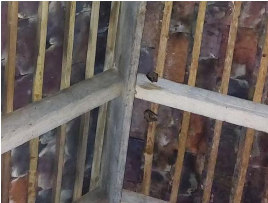
Plate 4: Close up of bats within the structure.
