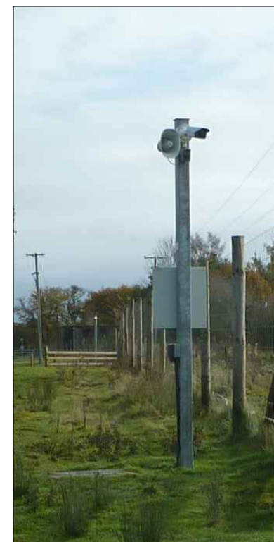
CCTV on adjacent site
