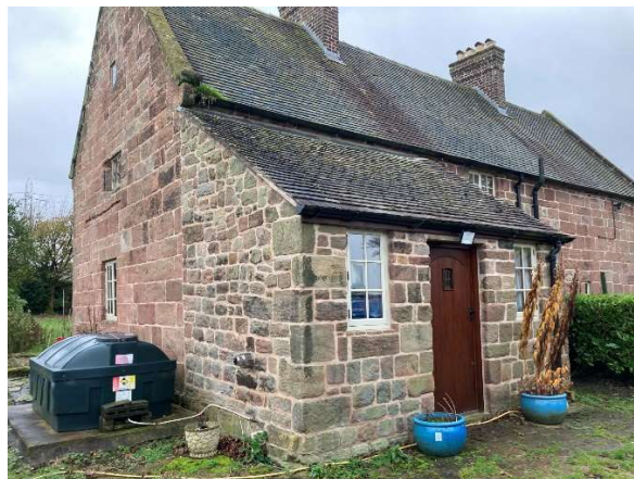
Image: Northeast corner of lean-to extension showing poor quality construction.
