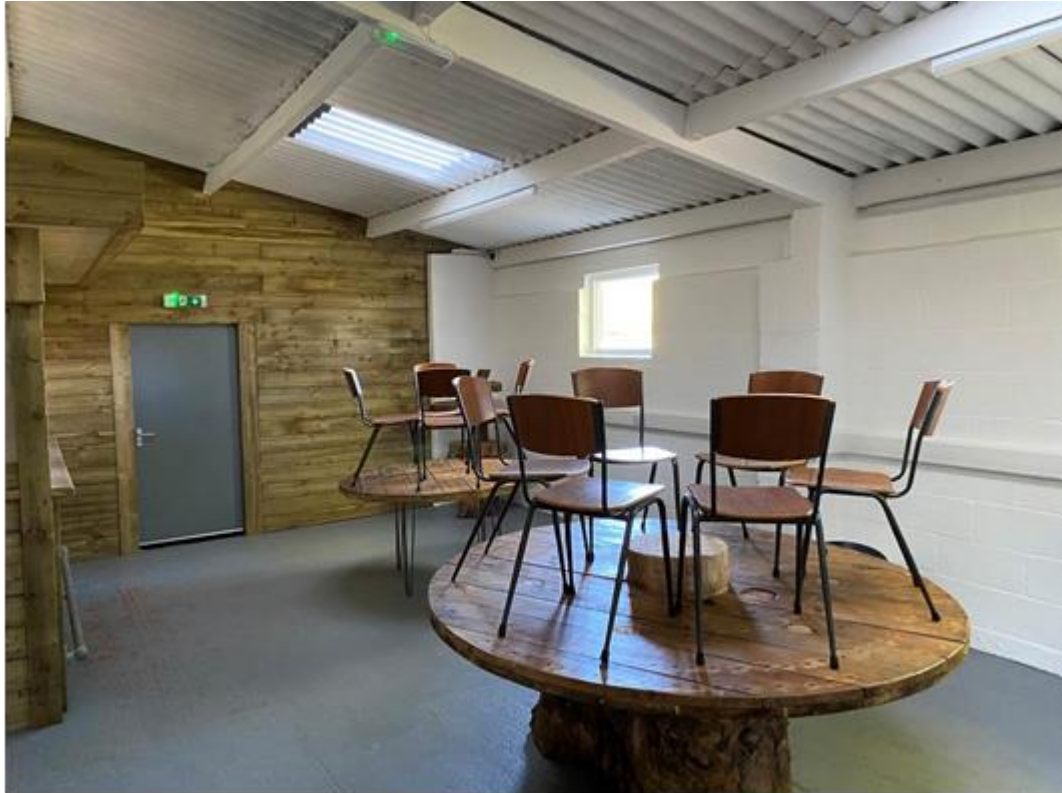
Figure 1: Image of venue prior to remedial works.
