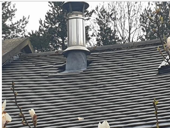
Plate IX. Gaps under common tiles around flue vent on south-eastern pitch of farmhouse.
