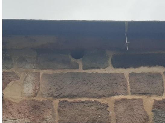
Plate VIII. Hole in stonework under eaves on north-western elevation of farmhouse.
