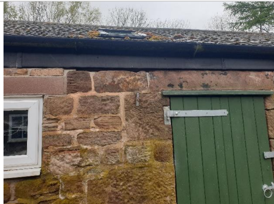
Plate V. Gap under fascia on south-eastern elevation of shippen.
