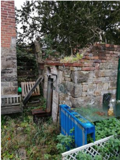
View 9: Stairs and adjacent pig sty
