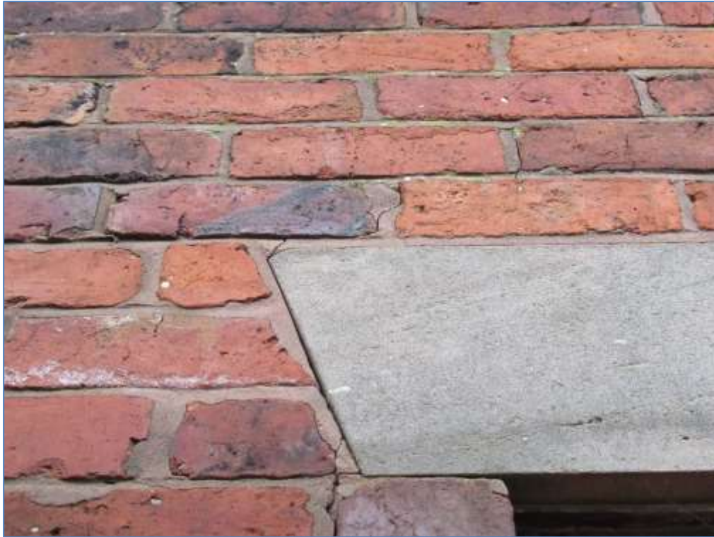
9. Shows cracking at the end of the lintel over the ground floor windows to number 82.
